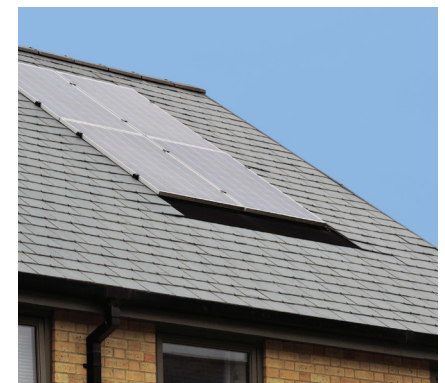
In-line solar panels
