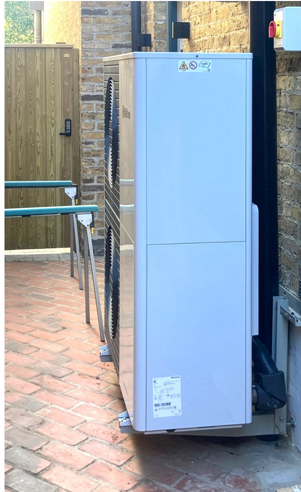
The air source heat pump (ASHP) sits discreetly along the side passage. Inside the basement, the system is supported by a hot water cylinder and an expansion vessel. The whole house is heated by low-temperature underfloor heating, which runs around 20°C cooler than a typical boiler, providing gentle, even warmth that works well with timber flooring.
