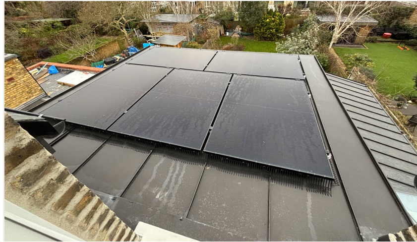
Photovoltaic solar panels on the two-storey rear addition zinc roof. In this location they have no visual impact
