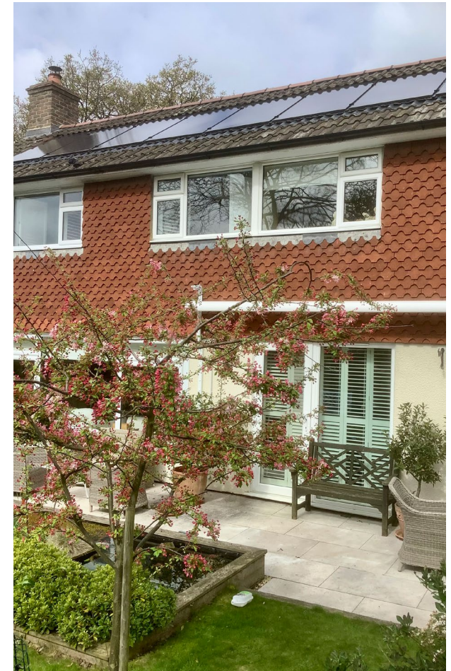
Roof-integrated solar panels to the rear roof
