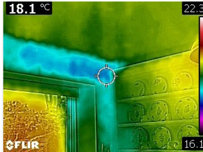
A thermal image survey shows heat loss through the lintel
