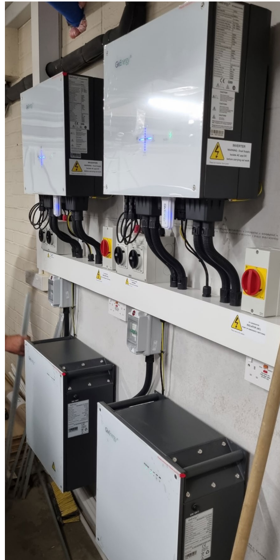
The battery storage is fixed to the wall of the garage
