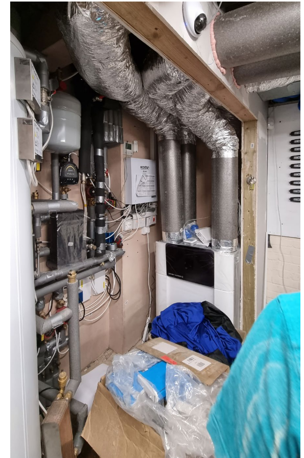
The MVHR system and hot water tanks are installed in the garage
