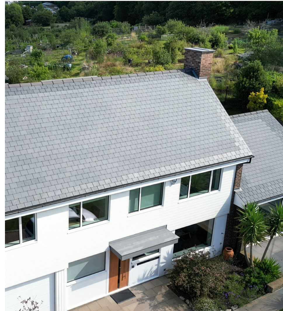
Replacing the roof enabled extra insulation to be installed and solar slates were added to the front south facing roof.
