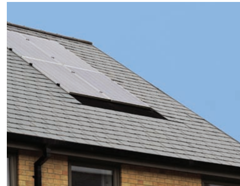
In-line solar panels
