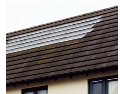
Integrated solar tiles
